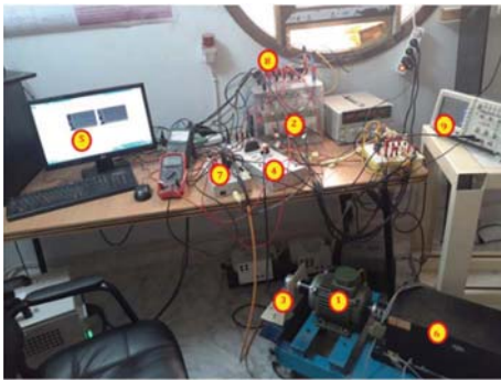
Fig.4 Test bench description.
